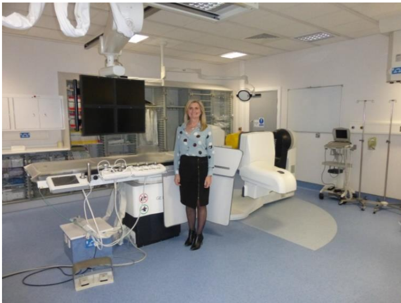
Gaile Smyth, Medipass MES Manager for Northern Ireland, with the Innova 540 interventional unit installed in September 2015.
